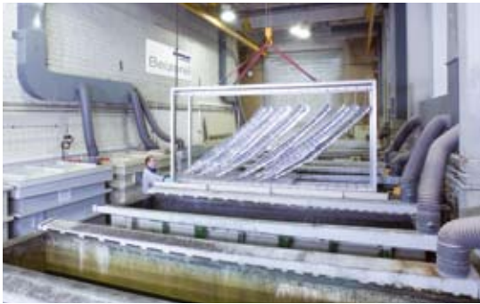
Pickling of aeronautical components at the Zeppelin galvanic shop approved by Premium AEROTEC.
